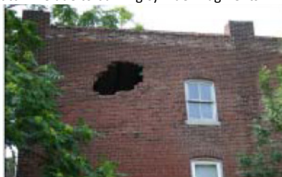
3-foot hole in side of residential building due to rocketing fragment, 530 feet away
