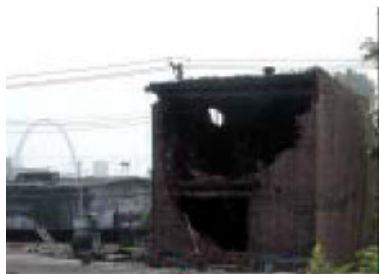
Burned out vacant commercial building, 300 feet away, from rocketing burning fragments
