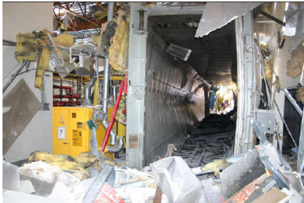
Sterilization chamber, after explosion
