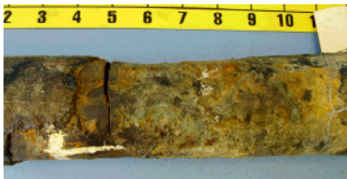
Cracked natural gas pipeline feeding house
