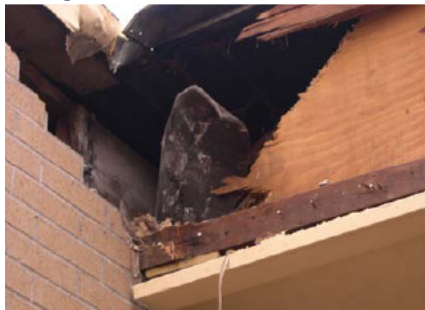
20-lb tank fragment embedded in a wall 300 feet from company property line
